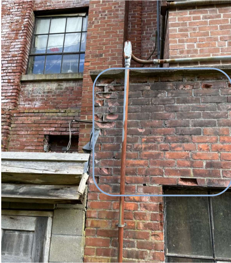
Figure 8 - Brick deterioration at the western face.
