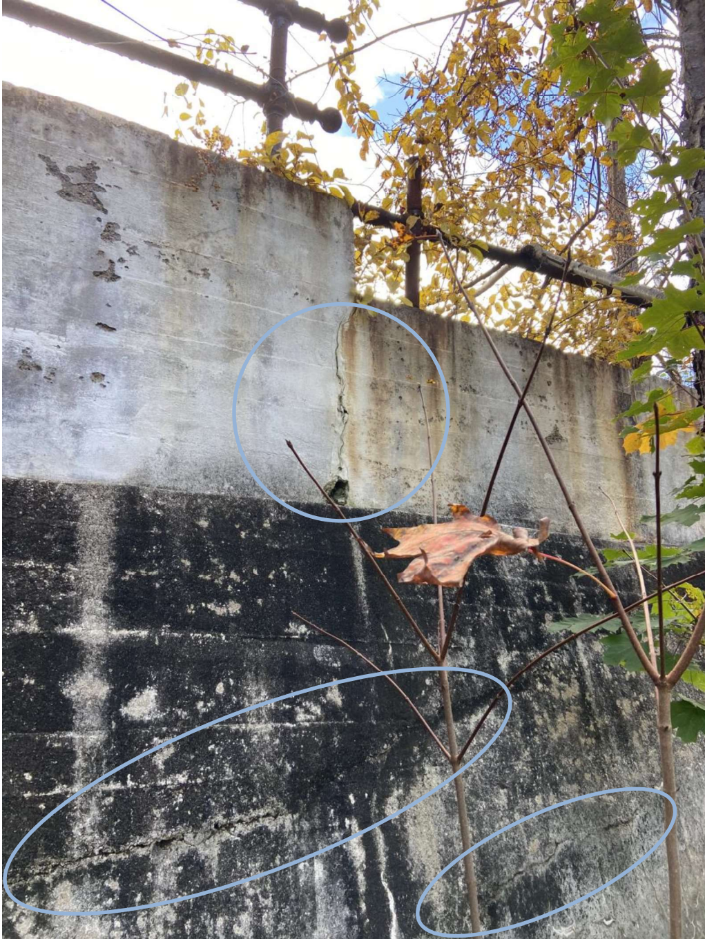
Figure 13 - Cracking in the concrete retaining wall.
