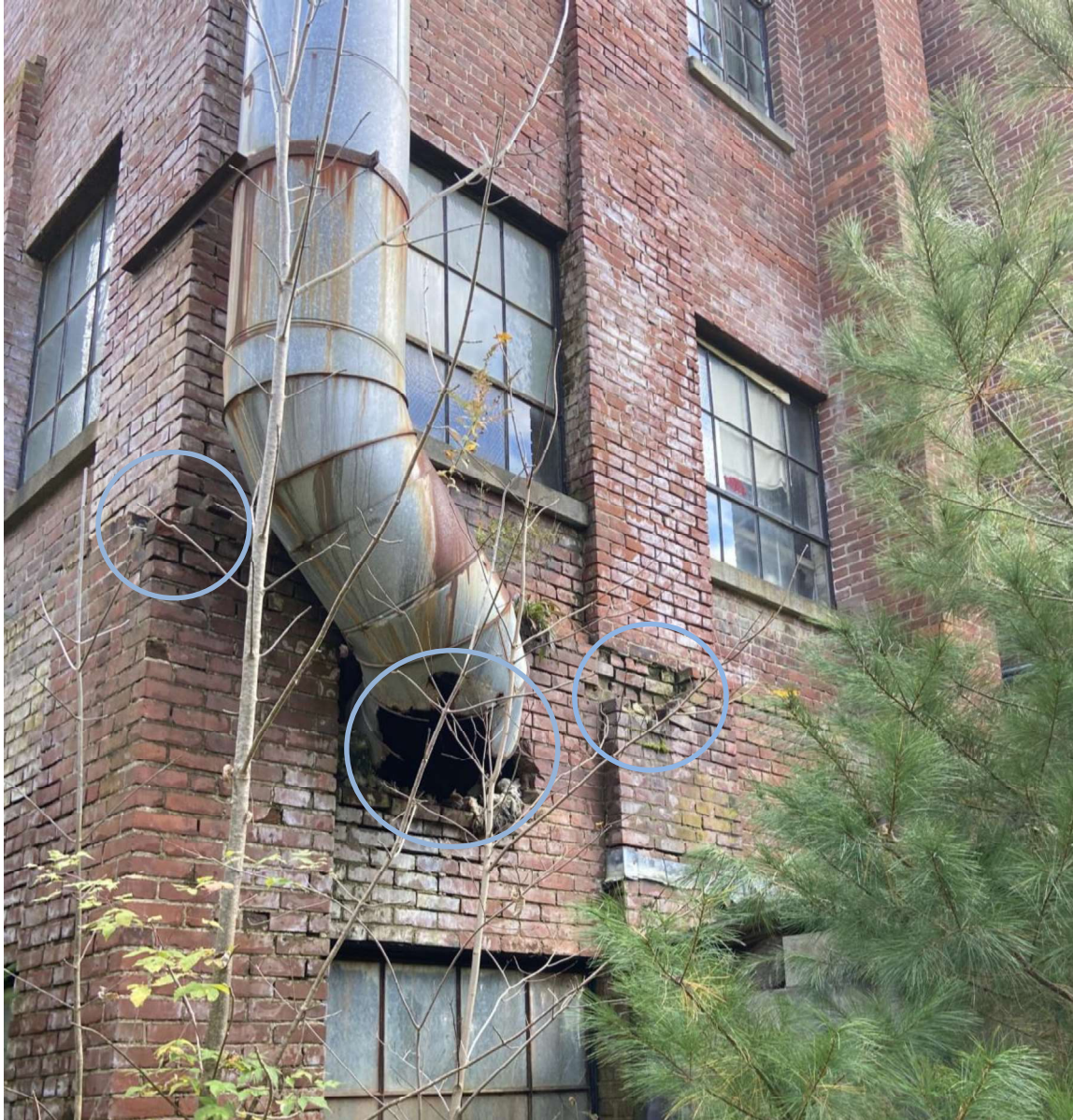
Figure 10 - Missing bricks at the NW corner.
