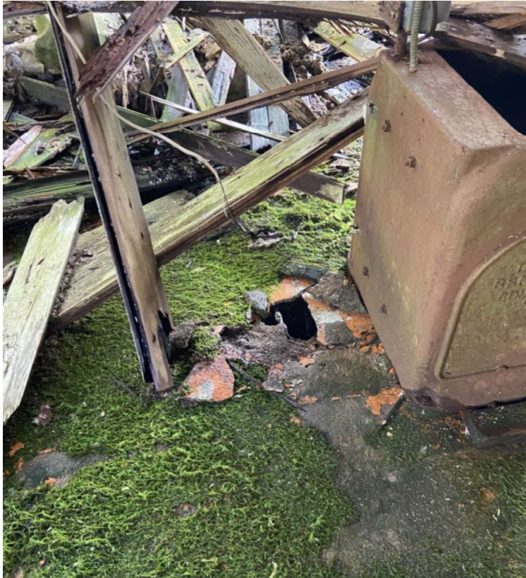
Figure 2 – Hole in the slab at the first-floor level.
