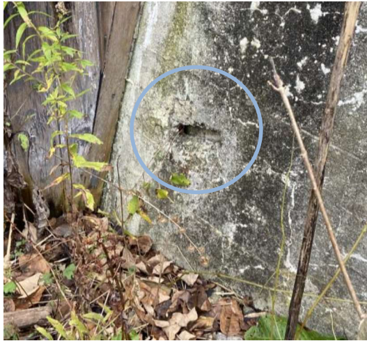
Figure 14 - Exposed steel reinforcing in the retaining wall.
