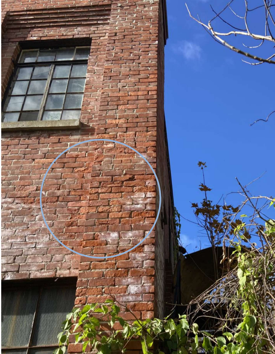
Figure 7 - Brick deterioration at the NE corner.
