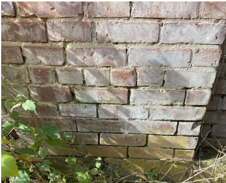
Figure 9 - Mortar loss and brick efflorescence.
